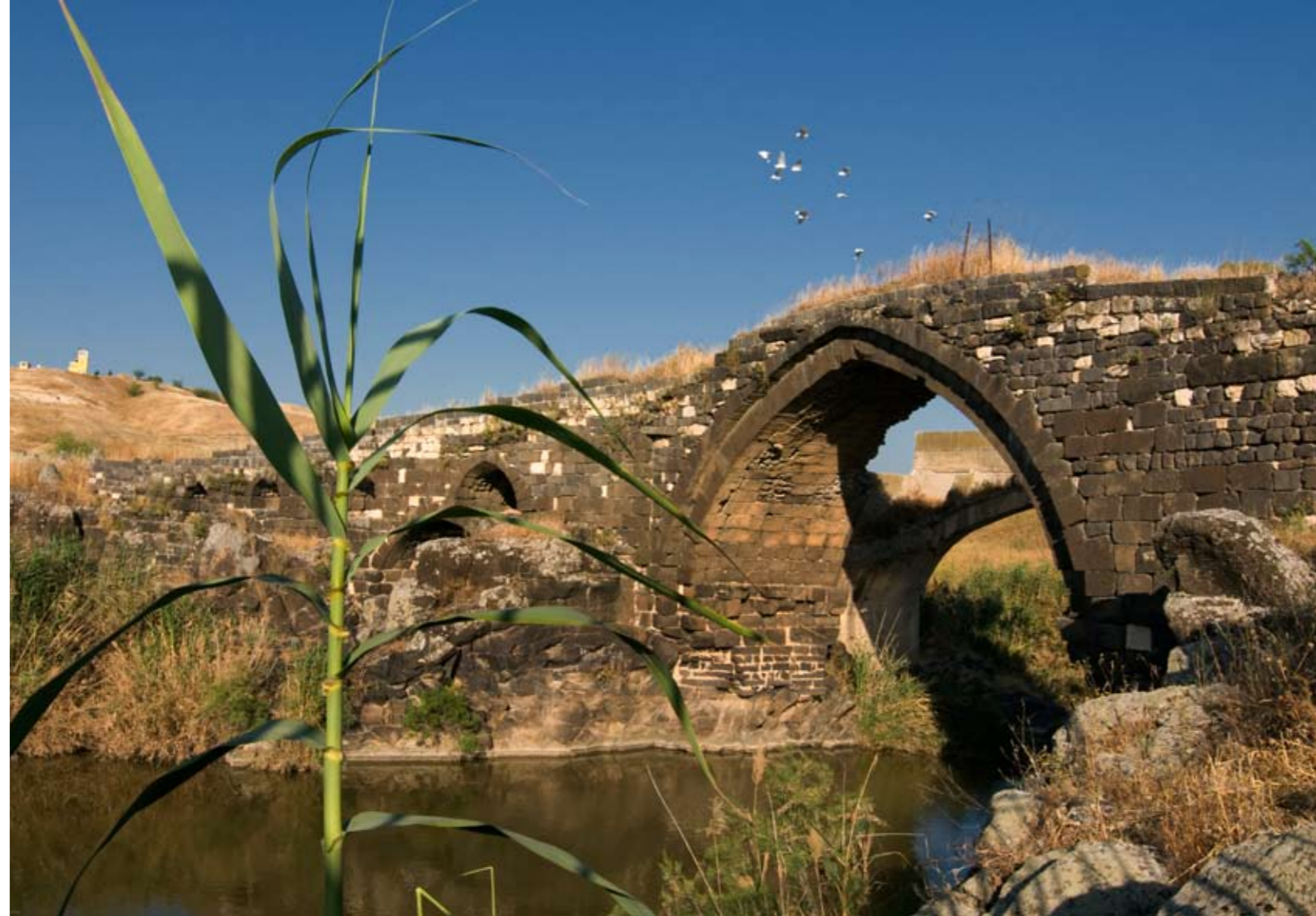
Three bridges traverse the Lower Jordan River including a 2000 year old Roman Bridge built from black basalt stones.
