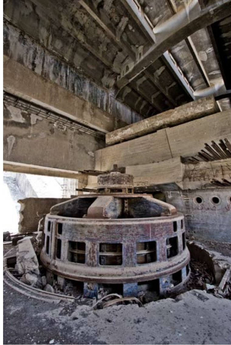
The interior space of the turbine hall was vaulted, clean and uncluttered, with the turbines set against a black and white checkerboard floor.
