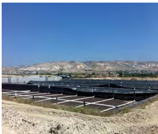
Figure 5: North Shouneh treatment plant, 2012, Photo: FoEME
