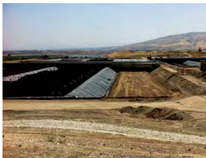
Figure 6: North Shouneh treatment plant, 2012, Photo: FoEME
