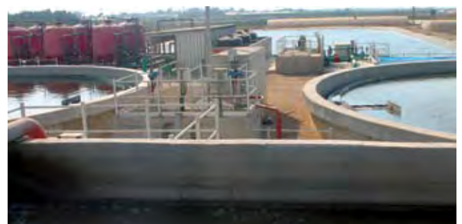
Figure 2: WWTP Baka Al Gharbia, Photo: FoEME
