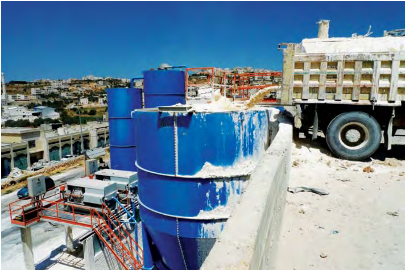
Figure 4: Truck disposing of stonecutting wastewater at Hagar Treatment Plant, Photo: FoEME
