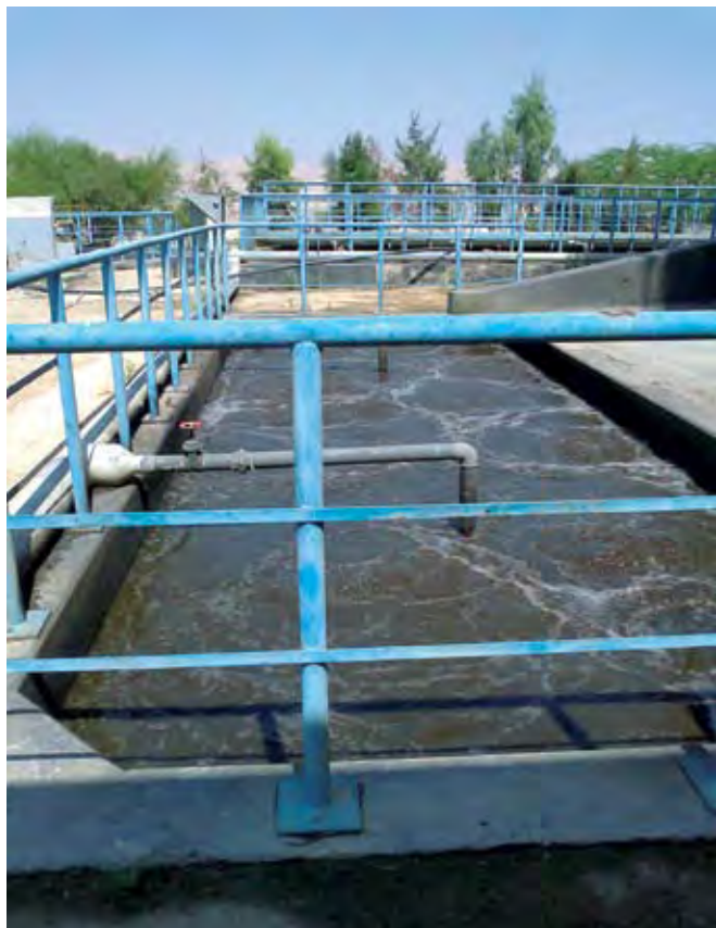
Figure 2: Tal Al Mantah treatment plant, August 2012, Photo: FoEME
