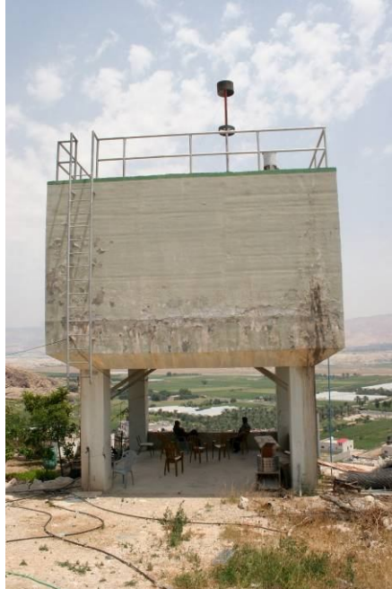
Water Reservoir in Az Zubeidat, 200 m 3 capacity. Photo: Jesse Baltutis
