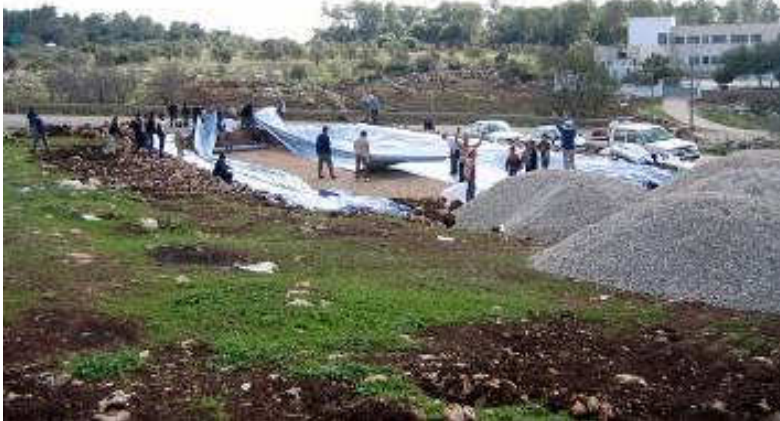
Residents build a natural filtration system for sewage treatment, Um Reihan (Palestine)
